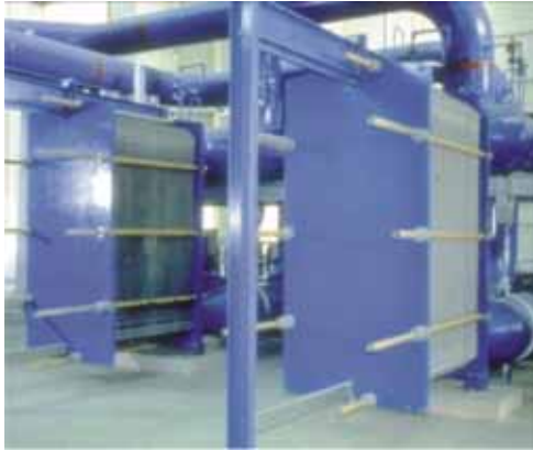
PHE was an unknown technology at the power plant.
